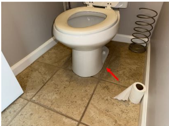
Toilet loose and may need re-anchoring. May cause leaking.
