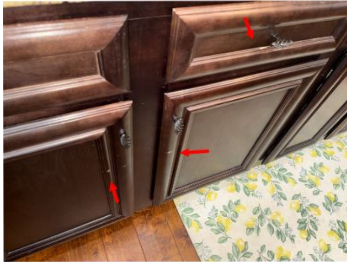
Minor wear damage at cabinets. Have addressed as needed.
