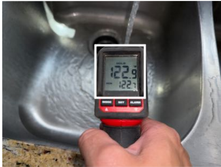
Water heater functional.
