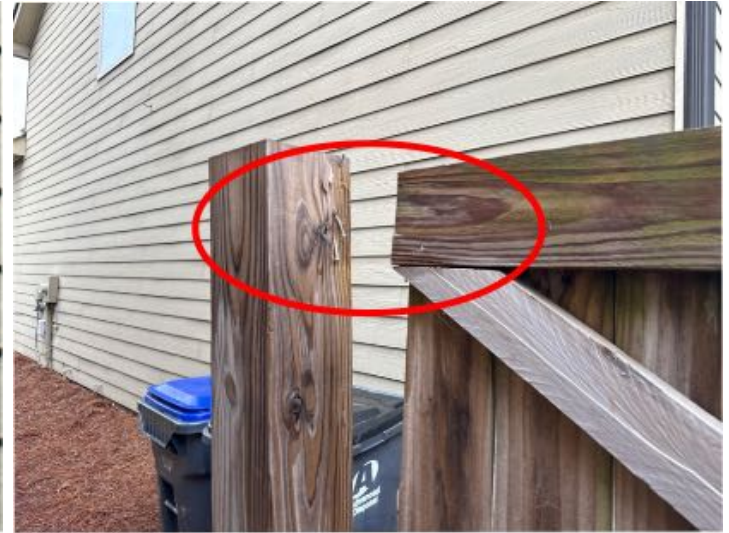
Gate not secured at right. Securing recommended for proper latch of gate without having to pick it up.
