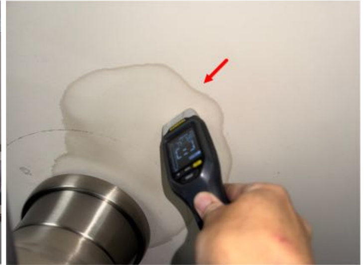
Water stain in front left upstairs bedroom ceiling. Tested dry at time of inspection.
