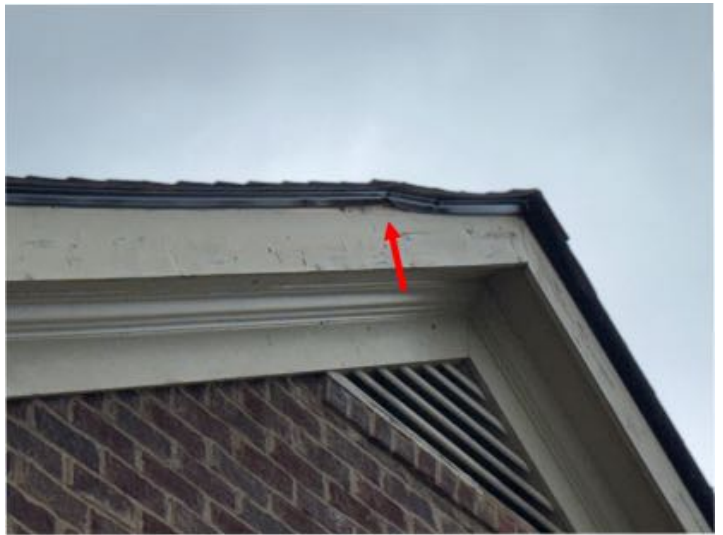
Minor damage at front center drip edge flashing. Repair recommended as this is meant to sit flush with fascia to help prevent water intrusion.
