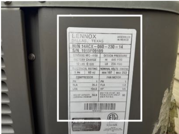
Data Plate: Lennox AC Unit: 2015 (11 years old); 5 Ton Unit
