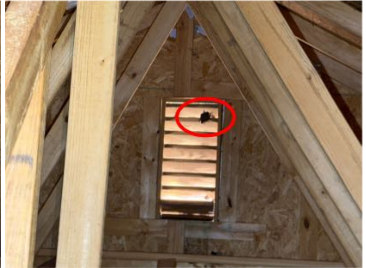
Bat noted at right gable vent. Pest control recommended.
