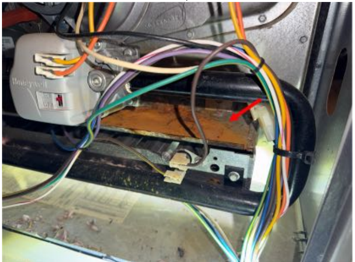
Minor rusting likely from condensation from drain line above. Monitoring recommended.
