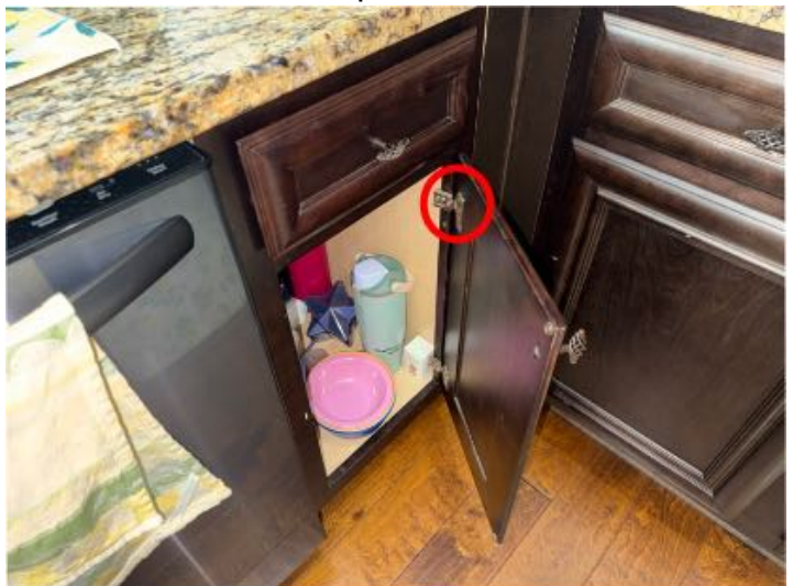
Cabinet door hinge loose to right of dishwasher.
