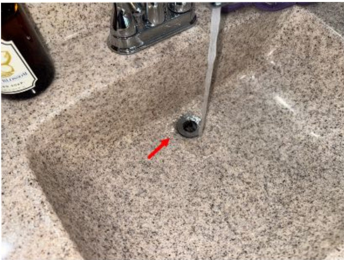
Right sink stopper repair recommended.
