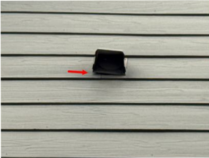
Bottom left of right front vent cover is not secured.
