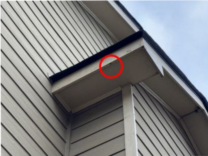
Possible carpenter bee damage at left center. Repair/sealing recommended.
