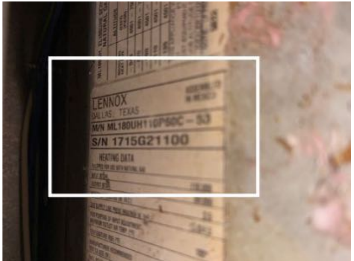
Data Plate: Lennox attic furnace: 2015 (11 years old)
