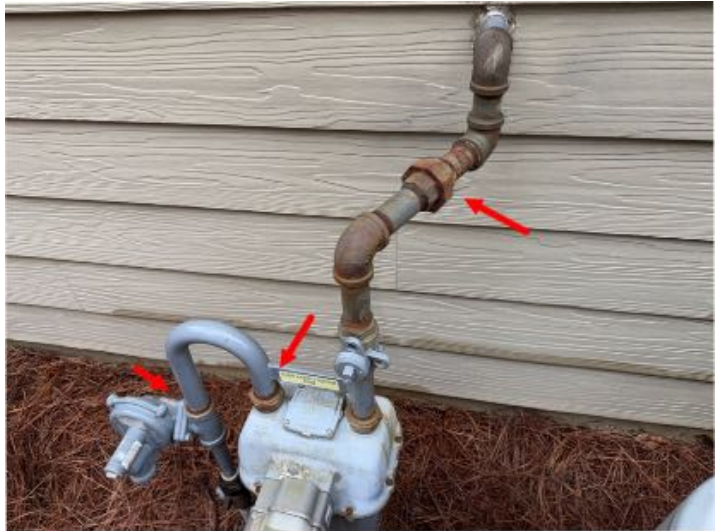
Areas of rusting noted at gas lines. No gas leaks detected at time of inspection. Consider sealing to help prevent further deterioration.
