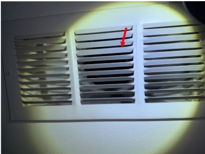
Dust buildup at return vents. Consider having ducts cleaned out.
