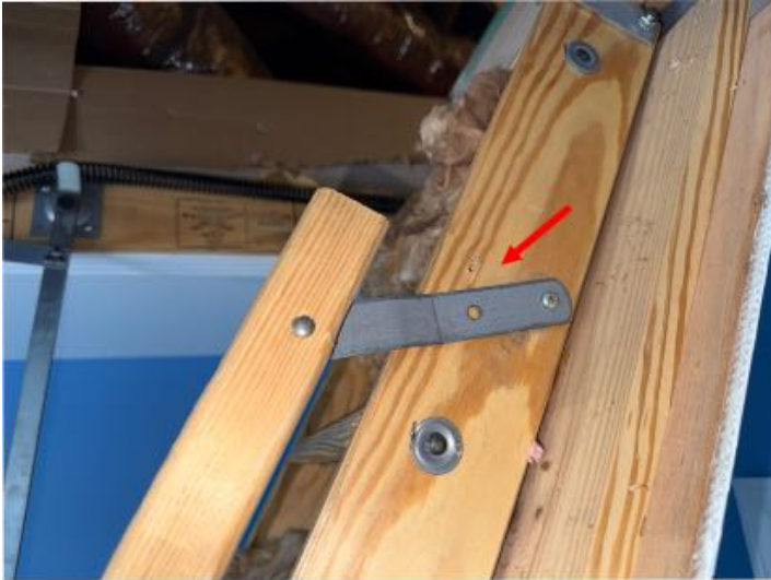
Securing attic stairs handrail recommended for safety concerns.
