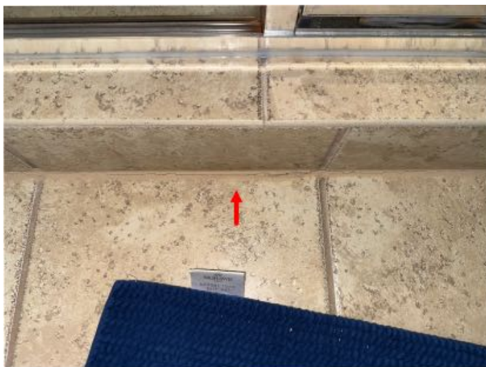
Tub/shower to floor junction missing caulk/grout. Repairs recommended.
