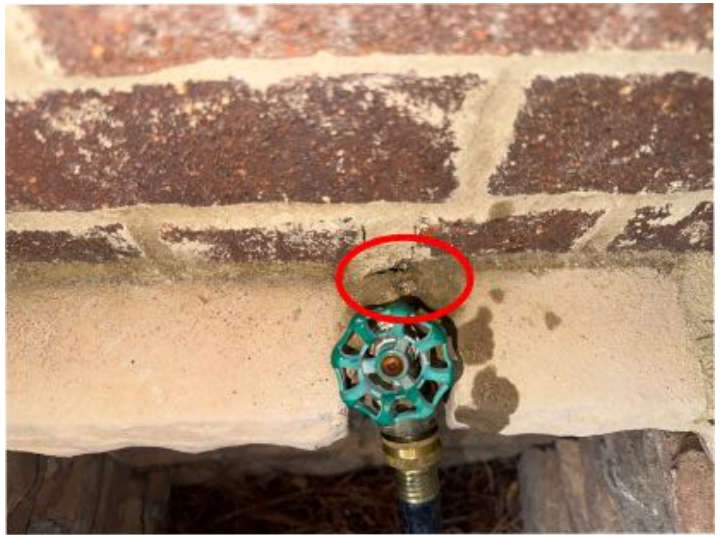
Hose bib has a gap at front center. All hose bibs be secured and sealed to prevent plumbing damage and water intrusion.
