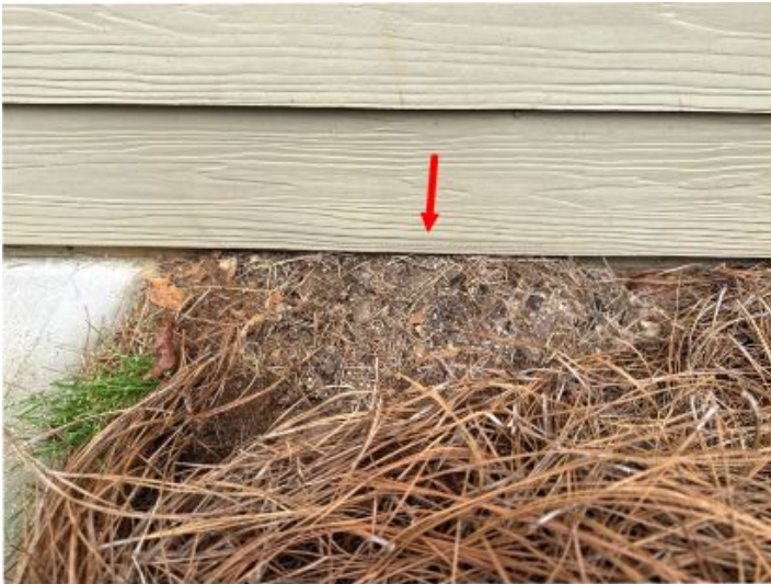
Siding to Soil contact. This can allow water or insect access to siding. Grading soil so there is at least 6" of space (where practical) between the siding and the soil recommended. Also, insuring there is no pest intrusion and damaged siding/trim recommended.
