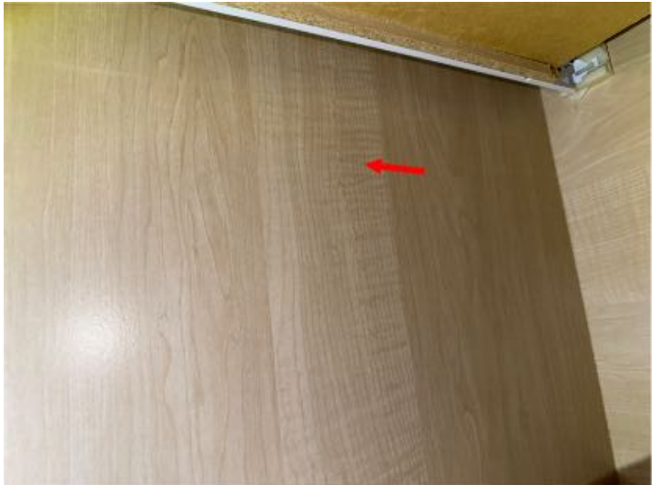
Left side of cabinet wall cracked. Have addressed as needed.
