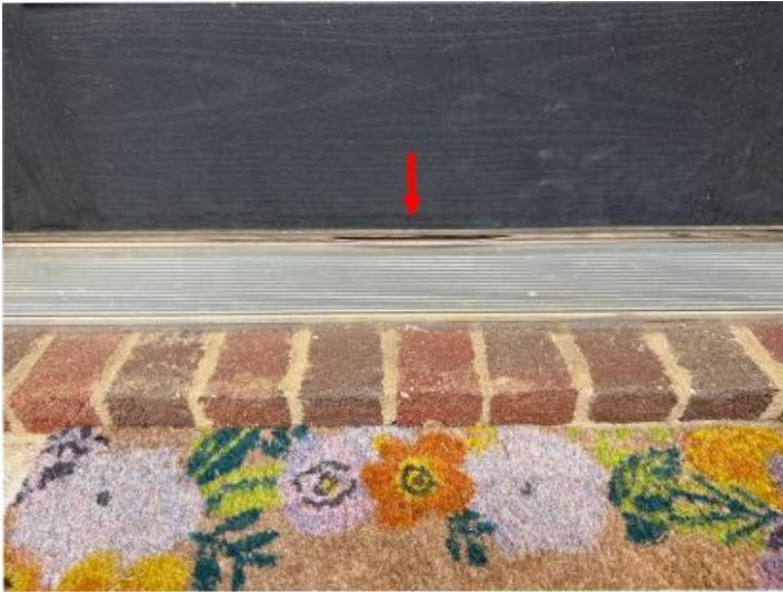
Minor weatherstripping damage at bottom of front door. Have addressed as needed for energy efficiency.
