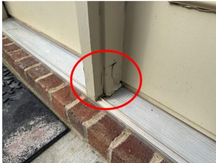
Wood deterioration/softening at rear door trim. Repairs and/or sealing (if applicable) to help prevent further water intrusion and deterioration recommended.
