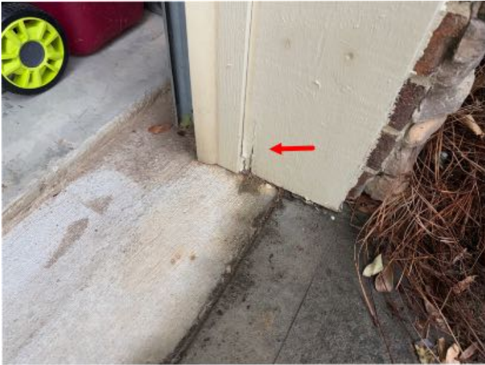
Minor trim damage at front right. To prevent further water intrusion and deterioration repairs and/or sealing (when applicable) is recommended.
