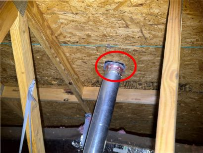
Gap at dryer vent connection to vent cover/roof sheathing. Resecuring recommended.
