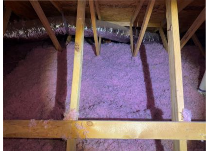
12 inch of insulation in attic. Insulation levels are specified by R-Value. R-Value is a measure of insulation's ability to resist heat flow. The higher the R-Value, the better the thermal performance of the insulation. The recommended level for most attics is to insulate to R-36/38 which is about 12/14 inches of fiberglass insulation.
