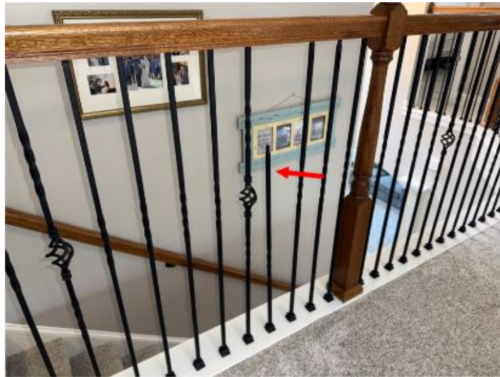
Spindle at top railing is too short. Repair recommended.
