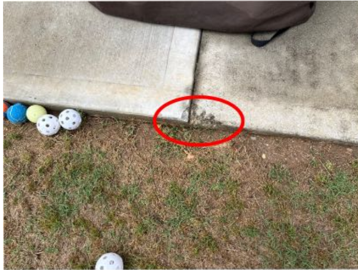
Minor damage at rear patio. Have addressed as needed.
