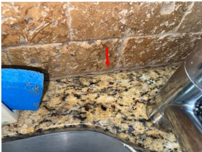
Sealant/grout at counters is deteriorating and/or missing. Resealing recommended.
