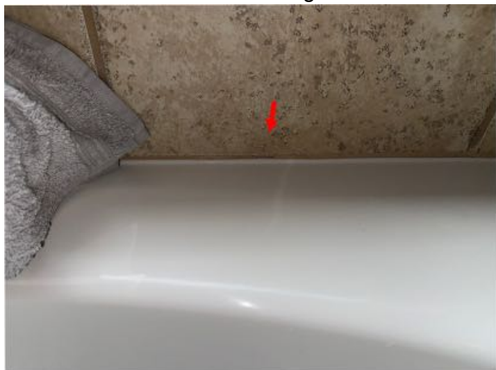
Sealant/grout at bathtub missing/deteriorating. Resealing recommended.
