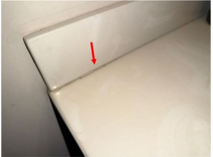
Sealant is deteriorating at sink counters. Resealing recommended.
