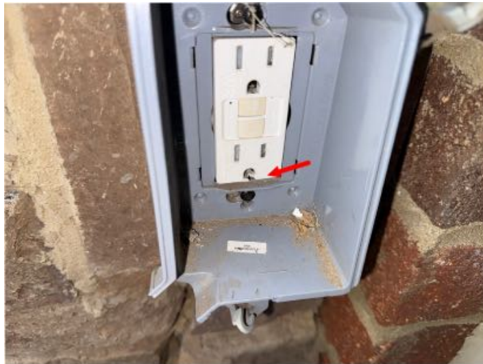
Minor damage at front center bottom ground of outlet. Have addressed as needed.
