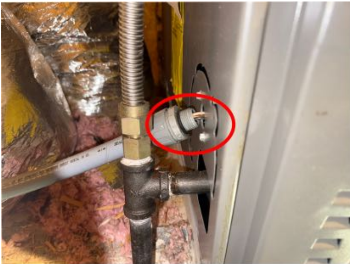
Resecuring conduit for electrical wiring at left side of furnace recommended to help prevent potential damage to wiring.
