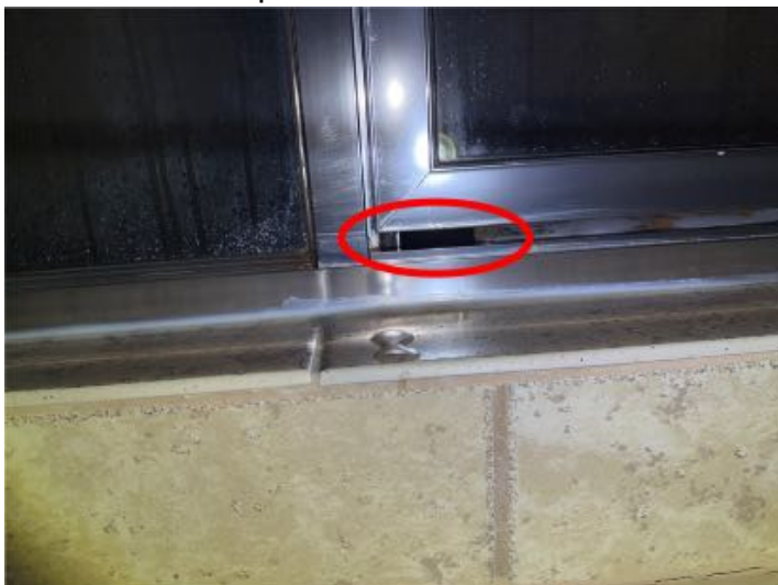
Minor weatherstripping damage at bottom of shower door.
