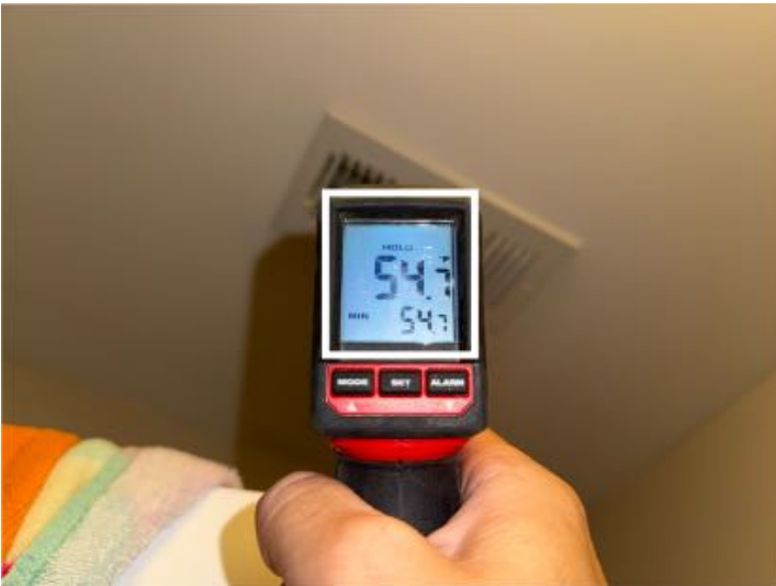
Upstairs AC tested good at 54 Deg
