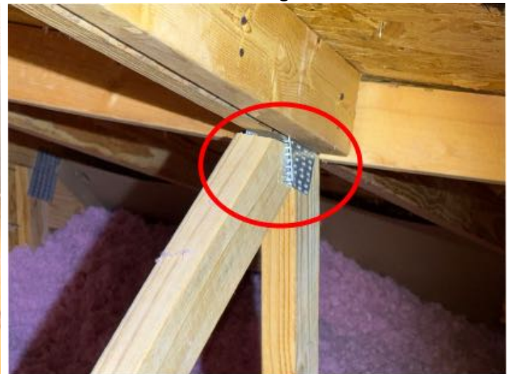
Nail plate is not secured to truss at rear left. Securing recommended.
