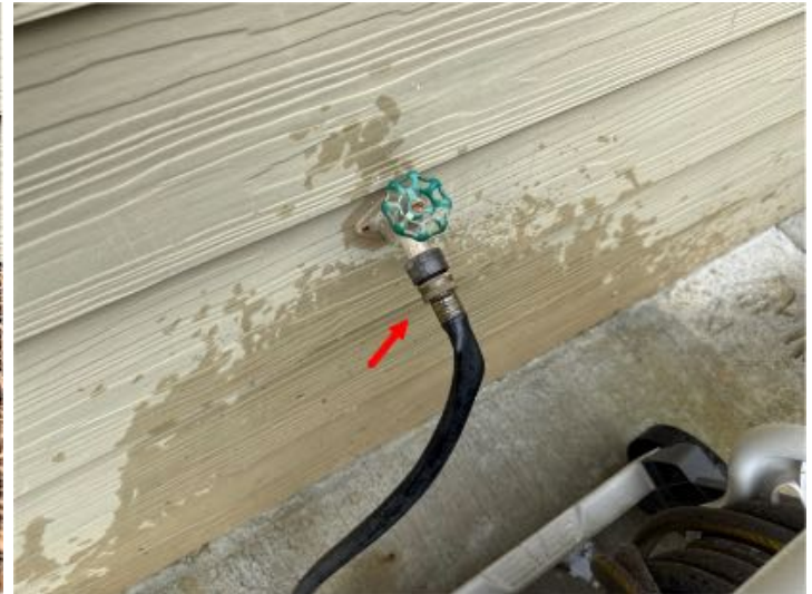
Could not get hose off of hose bib at rear right.
