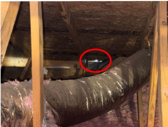
Gap noted in attic at front center. We recommend that this be sealed to prevent pest intrusion.
