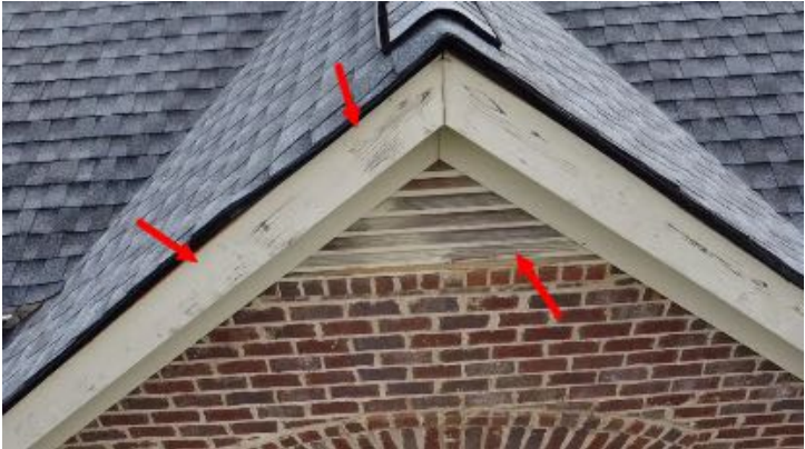
Minor fascia and trim damage at front center. To prevent further water intrusion and deterioration repairs and/or sealing (when applicable) is recommended.
