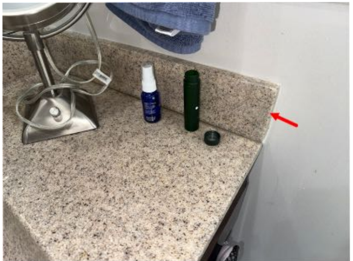
Sink countertop backsplash has some movement. Resecuring as needed recommended.
