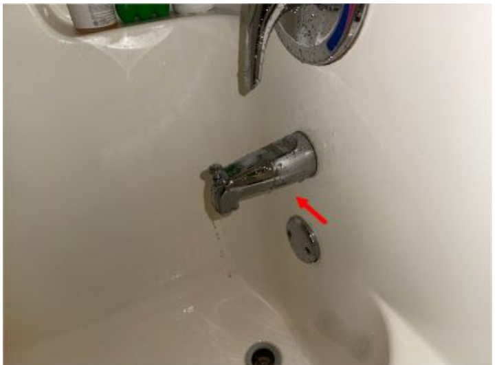
Tub faucet has some movement. Use caution and/or have resecured.
