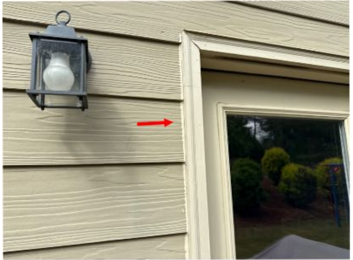
Sealant at rear center door trim has cracked. Resealing to help prevent further water intrusion and deterioration recommended.
