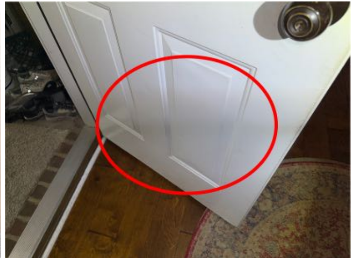
Minor denting at garage door. Have addressed as needed.
