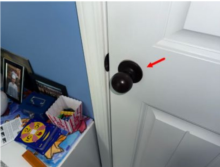
Multiple doorknobs loose throughout home. Resecuring recommended.
