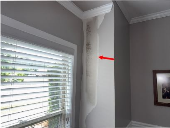
Minor damage at front right main level room wall. Repair recommended.
