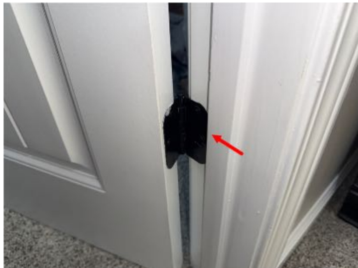
Bottom hinge loose at rear left upstairs bedroom door.
