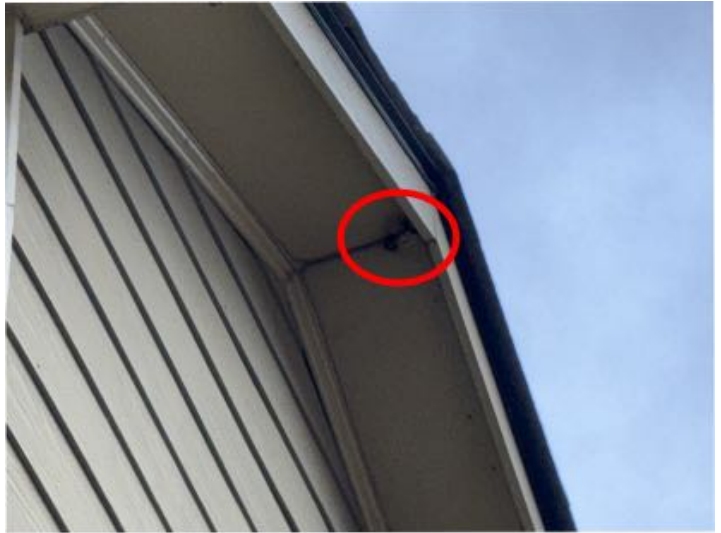
Stinging insects/nests at exterior. Pest control contractor recommended.
