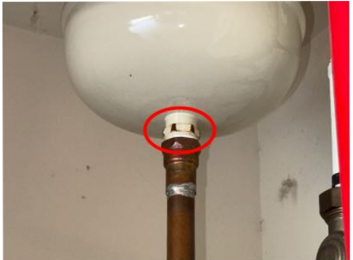
Minor rust noted at expansion tank. Monitoring recommended.
